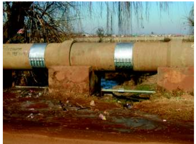
Above: The pipe after the quick response of the Metsi-A-Lekoa Maintenance Team.
